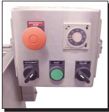
PLC BASED CONTROL PANEL
